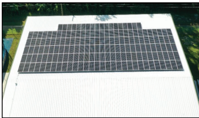
Solar Panels – Ruskin Recreation Center
