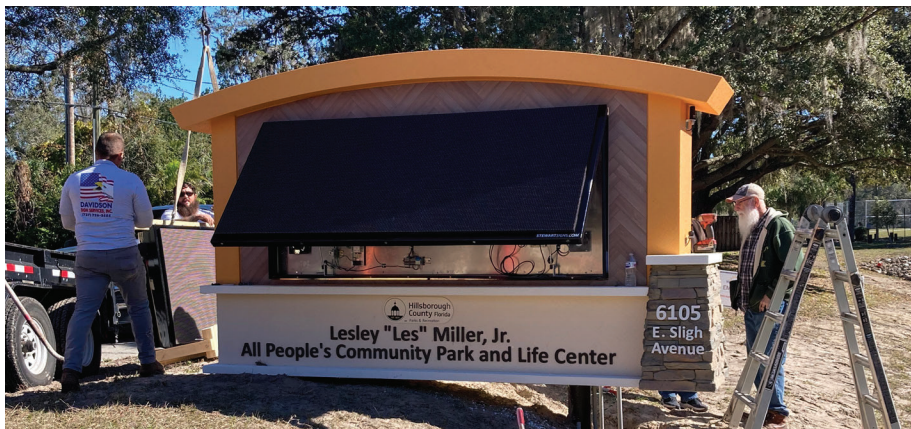
R3M installs the new entrance sign at Lesley "Les" Miller, Jr. All People's Community Park and Life Center.
