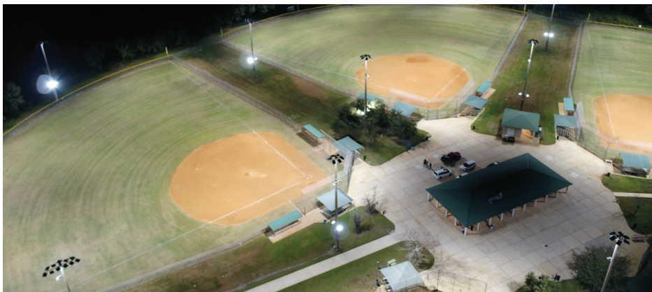
Newly installed energy efficient LED lights shine over the Ed Radice Sports Complex.
